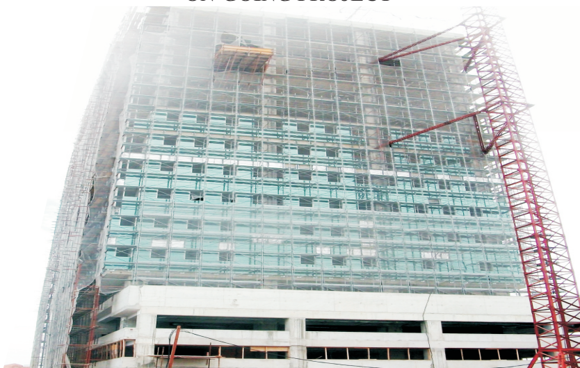
On-going Civic Centre Towers Project at Ozumba Mbadiwe Avenue, Victoria Island, Lagos
